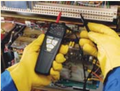
In voltage measurement, standard D2 test probes reach to the back of terminal strips.
